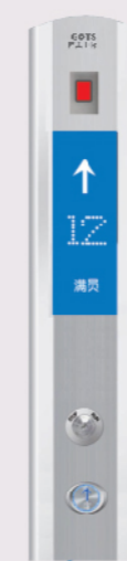
TS-W01 Integrated call and fire fighting panel at the first-floor base station (embedded)
